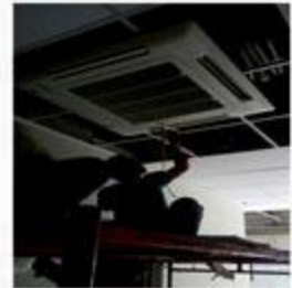
AC SPLIT DUCT
