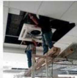
AC SPLIT DUCT
